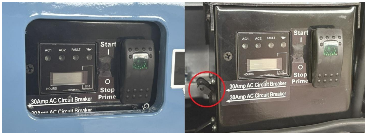
Figure 116. NPS Generator exterior control panel on the face of the generator with the cover on (left) and with the cover removed (right) showing the location of the line resetting circuit breakers.
