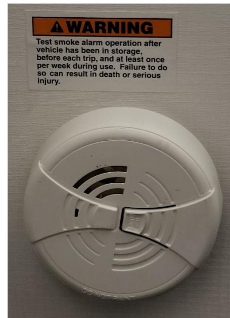
Figure 26. Ceiling mounted smoke alarm.
