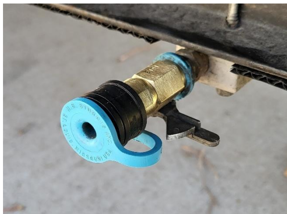
Figure 31. External propane quick connect, with flow lever in the "off" position.
