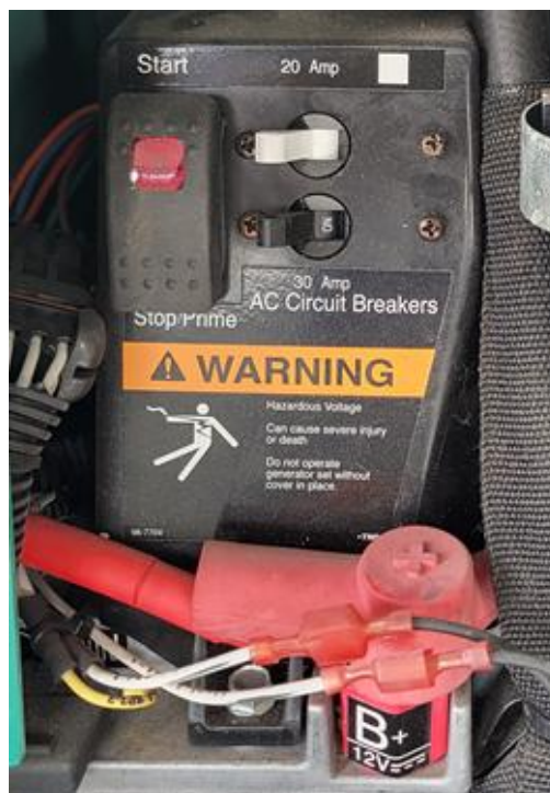
Figure 118. On-board controls for the Onan 5500 generator. The start/stop button and integrated fault light are on the left, and circuit breakers are on the right.
