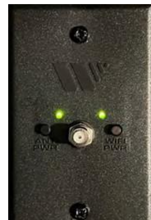
Figure 120. Winegard booster switch, with booster and Wifi enabled.
