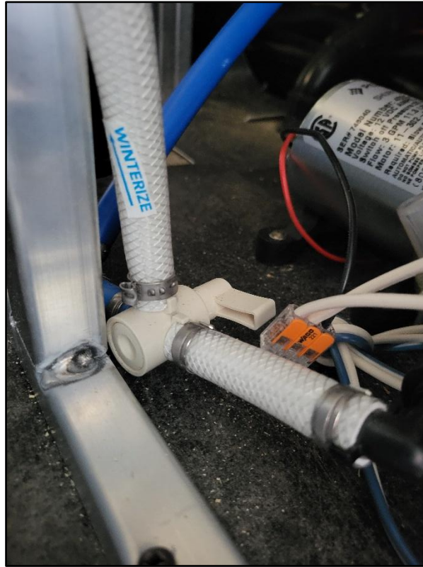
Figure 149. Winterizing diverter behind the main panel. This valve in this orientation will pull water from the fresh water tank to supply the water pump. Rotating the valve up will allow the water pump to pull fluid through the connected hose- usually placed into a container of antifreeze for winterizing.
