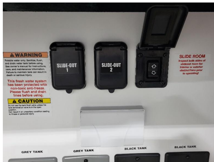
Figure 36. Remote slide controls in the utility bay of the Valor.
