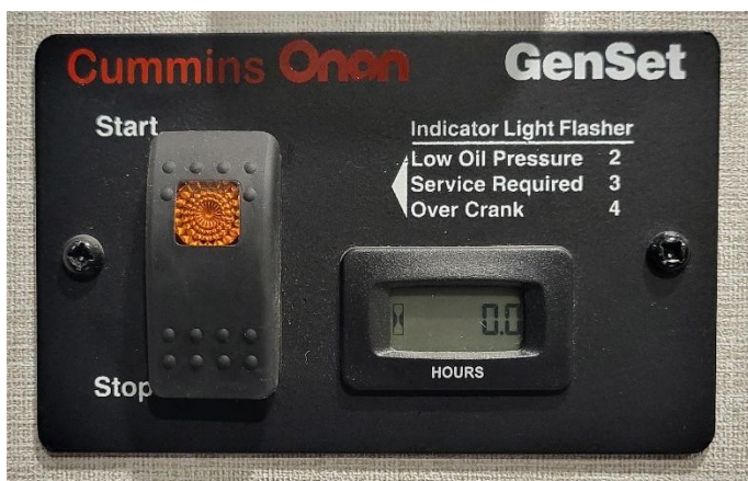
Figure 117. Remote generator start panel. The start/stop button and integrated fault indicator are on the left, and hour meter on the right.
