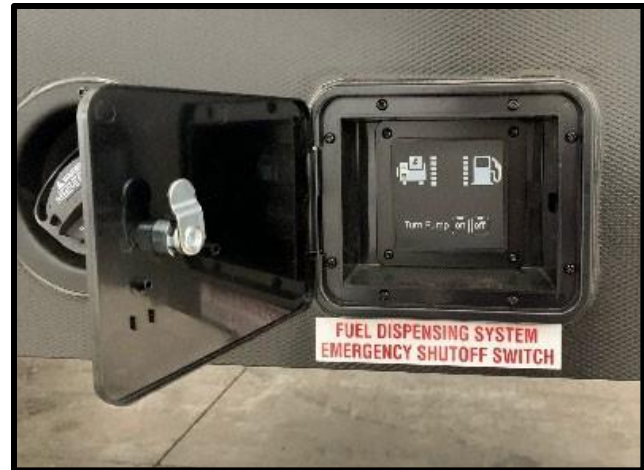
Figure 138. Fuel station control panel in sleep mode.
