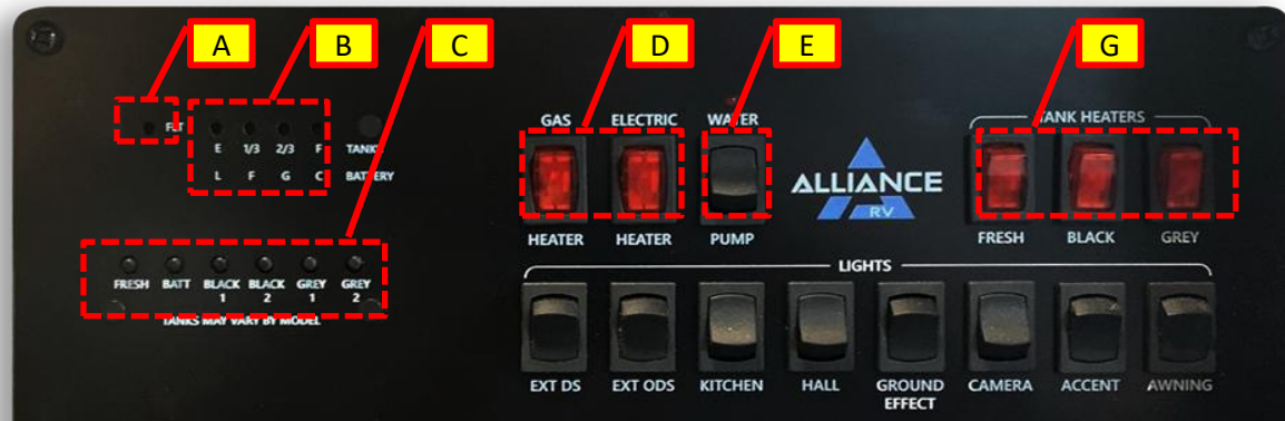
Figure 158. The upper portion of the monitor panel showing tank and water controls. This figure has the same indicators as Figure 122.
