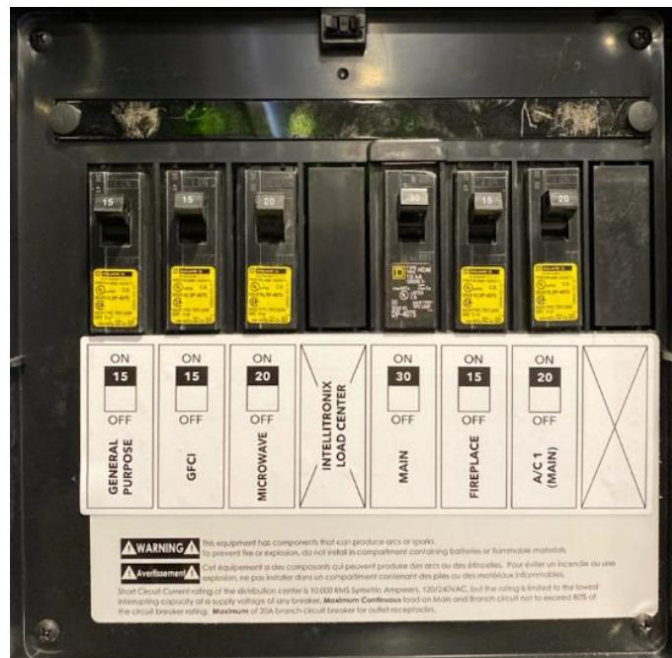
Figure 78. Intellitronix power module details.
